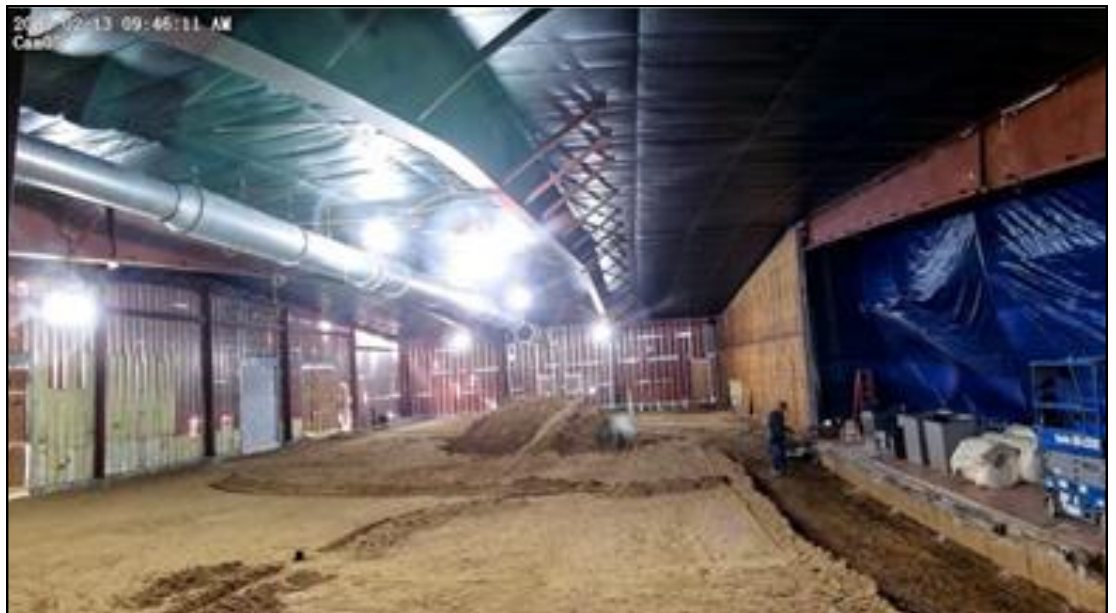
This photo shows the floor of the expansion being readied for concrete installation.
